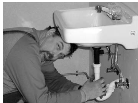
Thanks to volunteer David Haworth for plumbing the new service building on the greenhouse complex.
